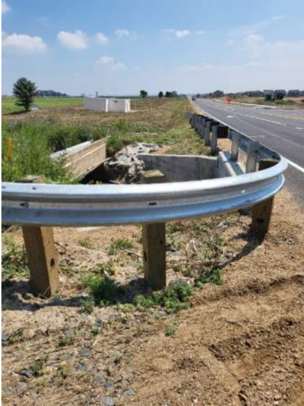
Guardrail needs to be secured and set
