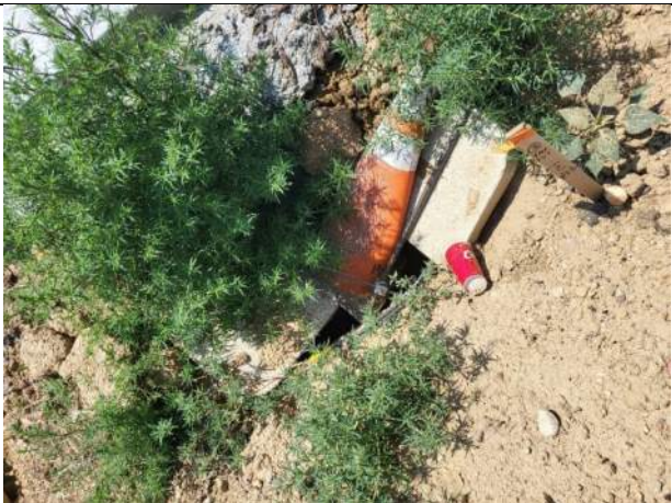
Utility Box low
